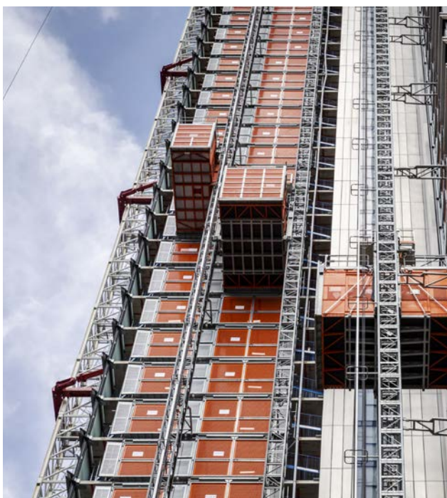
Alimak High Speed and Mammoth hoists at the South Quay Plaza in London, UK.
